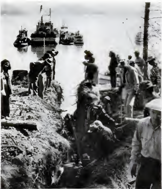
ANCHORED TO SHORE , cable is played out from the barge as it moves away from land. Ditch leads to powerhouse set up in anticipation of big event.
